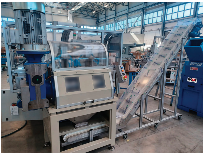
Shredding Extractor conveyor belt
